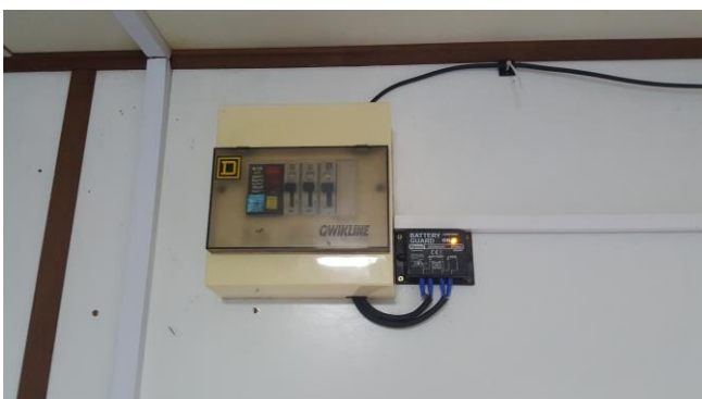
This is Mat's installation of the Under-Voltage Protection device. He admits that he might not have read the instructions (Mat Dawson photo).
