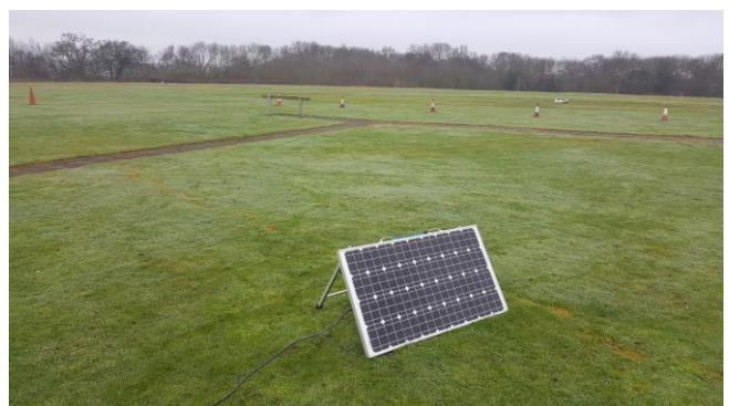
This is where the Solar Panel needs to be placed (Mat Dawson photo)...
