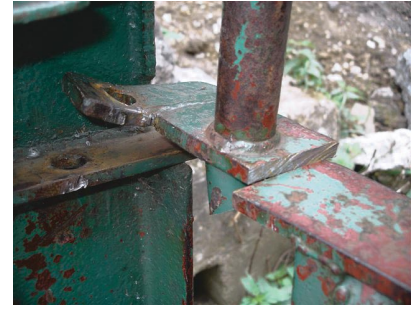
Damage done by hacksaw and crowbar.
