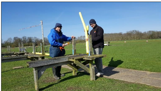
Mike Pugh and Mike Marman formed an impromptu work party to replace the buffer padding on the model benches
