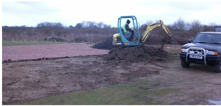
Roger hard at work excavating the muddy area of the car park next to the gravelled area which will be covered with scrapings
