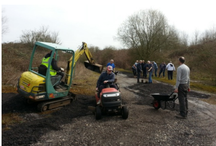
Roger with the mini digger filling Des's trailer with another load of scrapings
